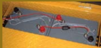
High Quality Gel Batteries No Maintenance, Refilling or Liquid Acids
